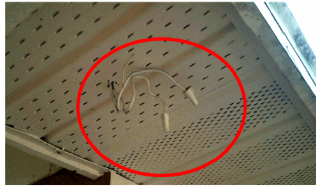
Exposed wires on Eave
