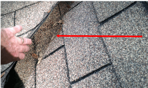
Another valley. Moisture under shingles. possible leak point
