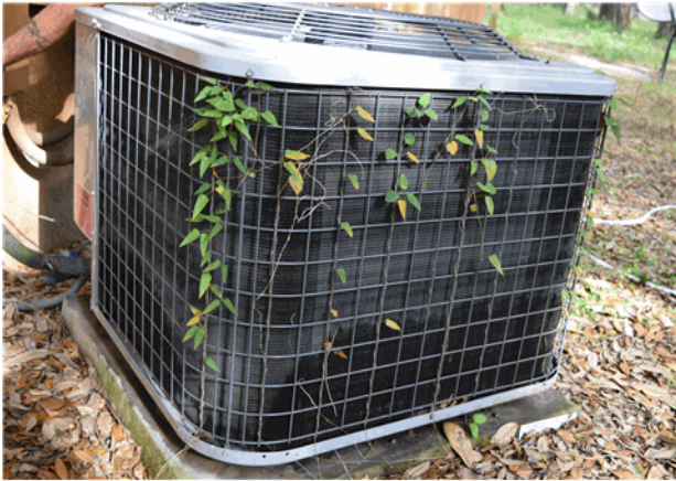
Recomend Maintenance on compressor unit of AC
