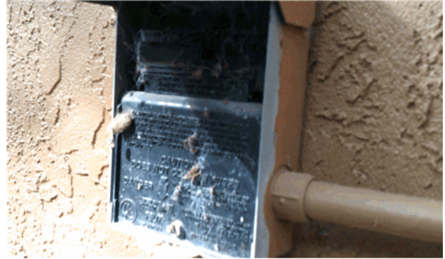
AC disconnect withing reach of unit
