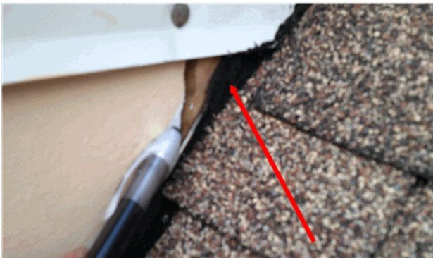
Not flashed. Opening to attic and trusses. Leak point
