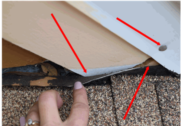
Exposed nail needs sealed. Exposed truss, not flashe properly at gable
