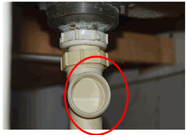
Wrong downspout from sink.
