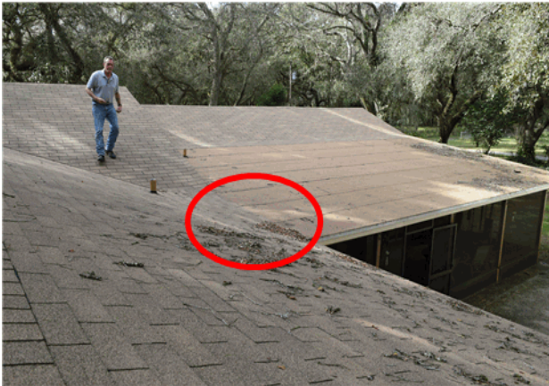
Area circles is less than 1:12 pitch and requires flat roof installation practice. Possible leak pt
