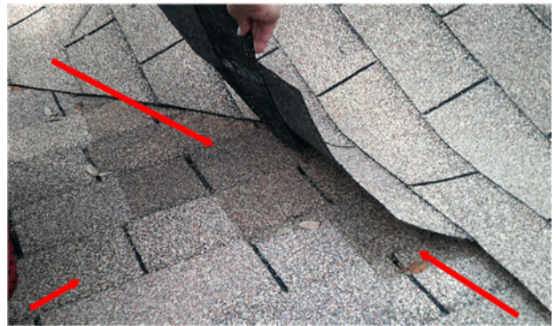
Improper Valley install. Picked up shingles.
