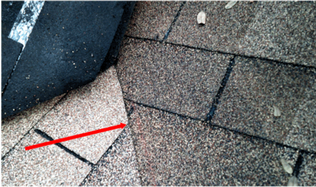
Another bad valley install. Picked up shingles
