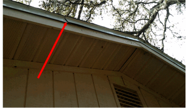
less than 1 inch over lap on drip edge
