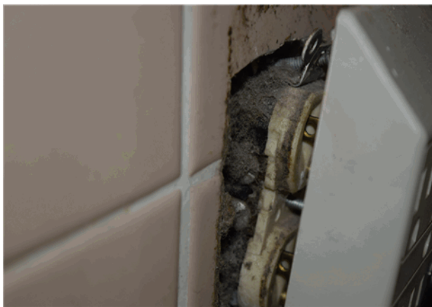
Kitchen outlet pulled out of wall
