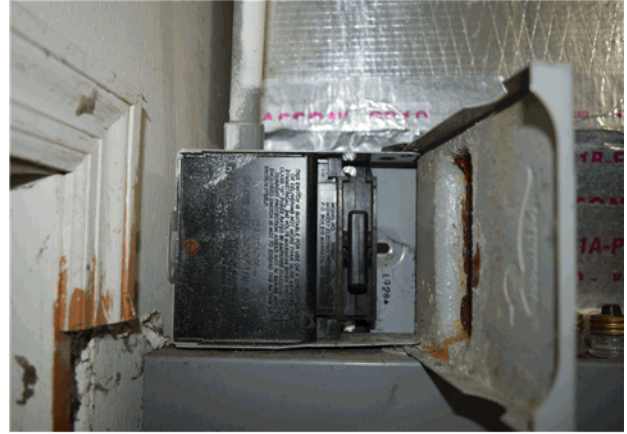
Air Handler disconnect switch. Unprofessional install
