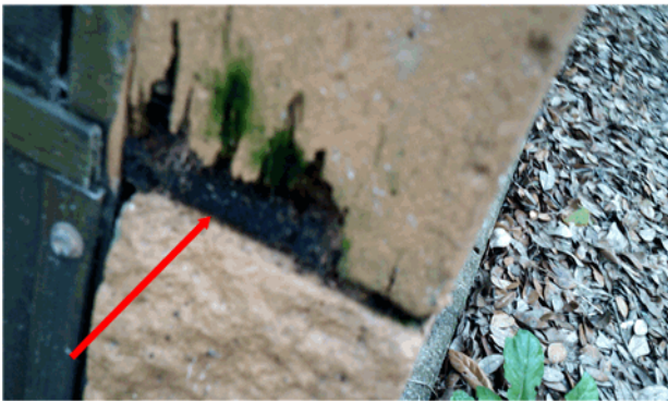
Patio wood rot on post
