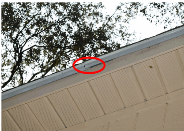
Drip edge not overlapped properly
