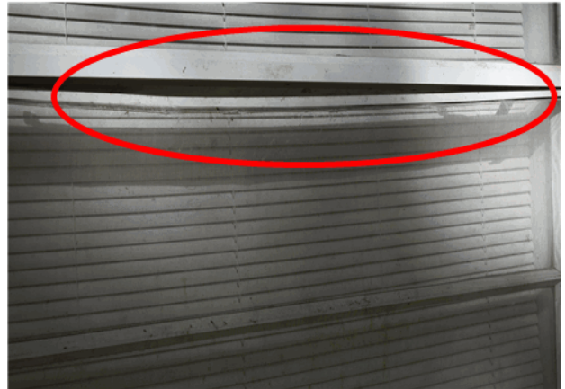
Damage Screens on most windows in home
